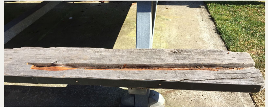
Photo documentation of damage 2017
