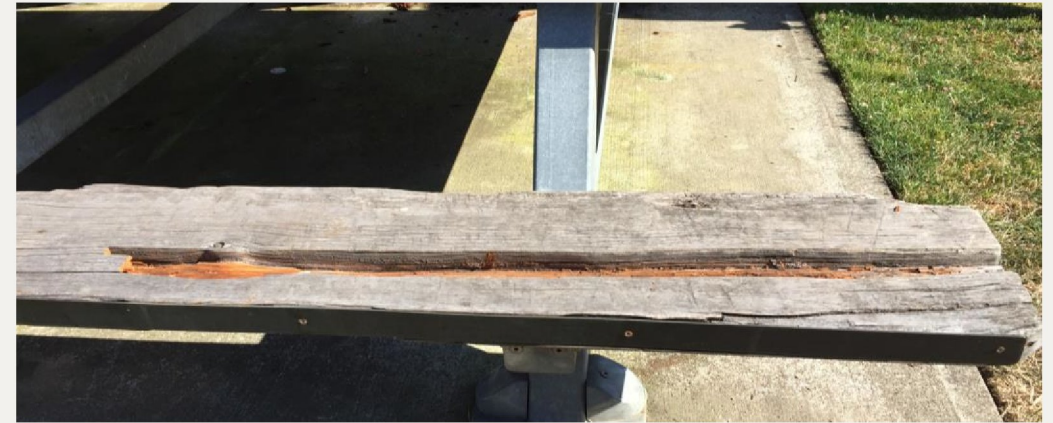
Photo documentation of damage 2017
