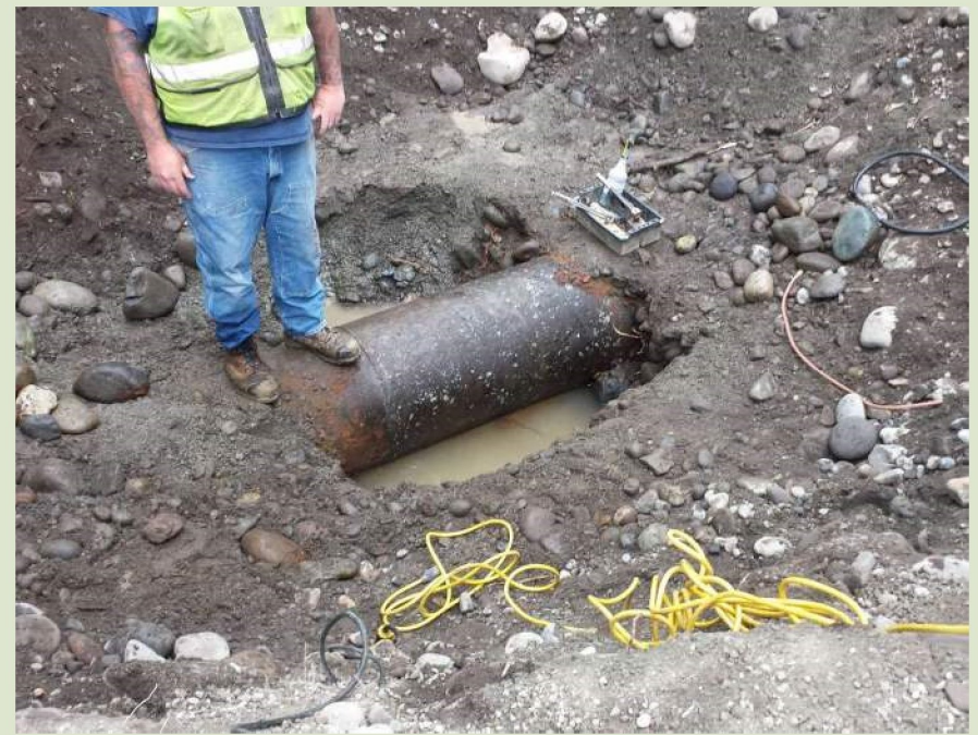
(Photo of nearly 100-year old transmission main)
