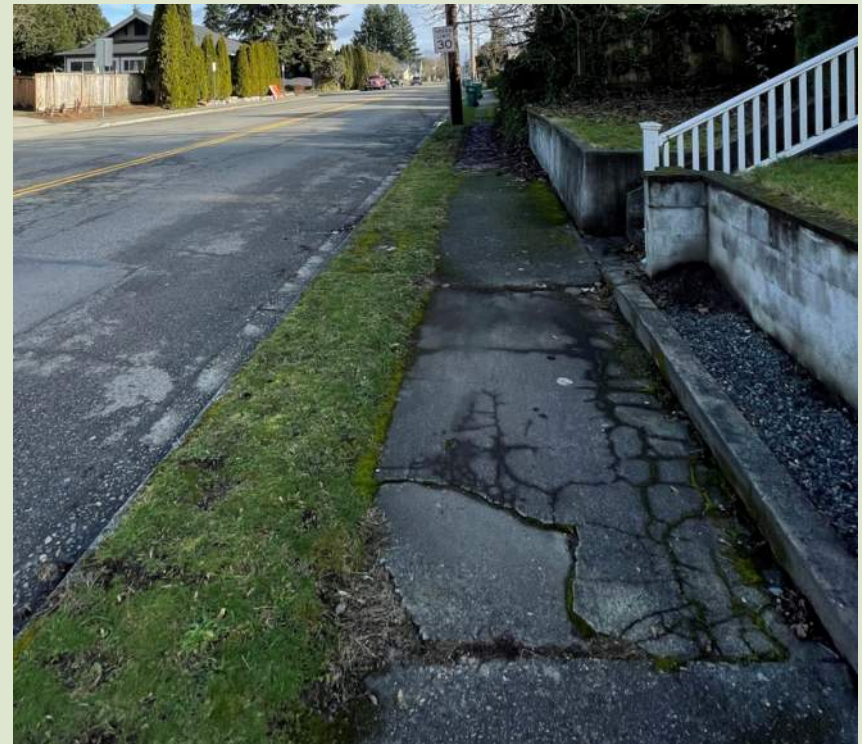
Right – Damaged Sidewalk.
