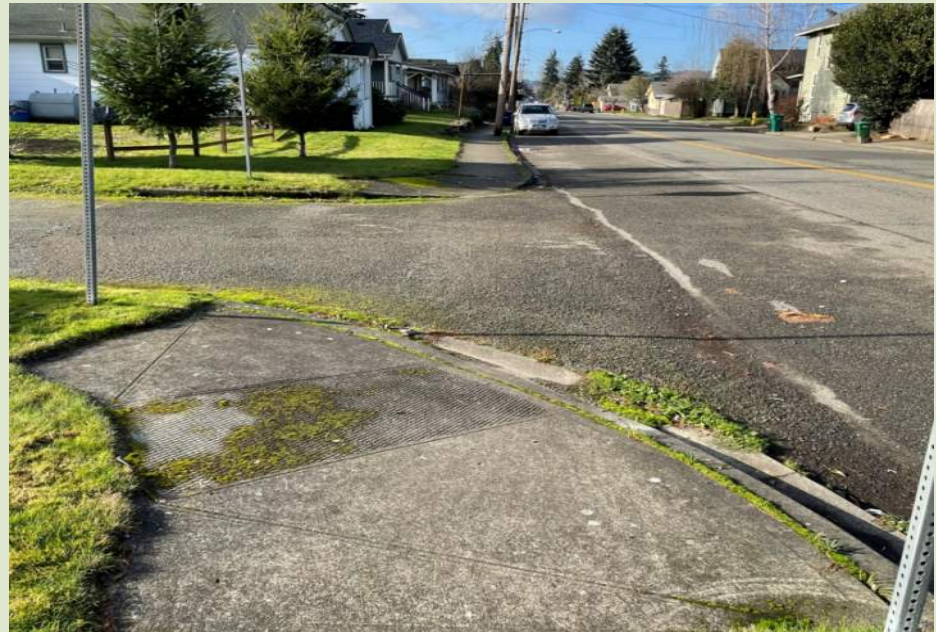
Substandard Curb Ramps
