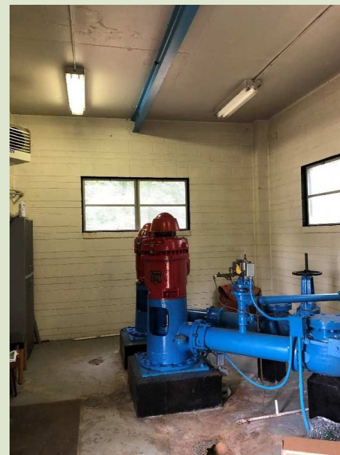
Pumps inside Pump Station 1
