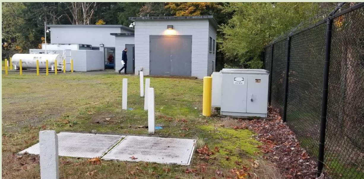
Academy Pump Station Facility
